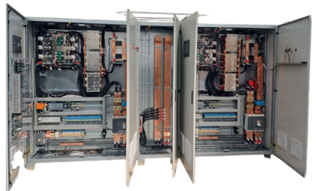
Internal View of SCR Dual Configuration
